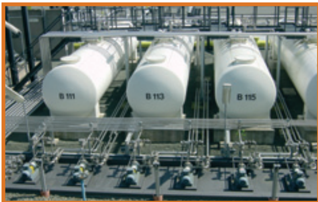
Pompaggio di additivi per olio lubrificante in Germania Pumping of lubricating oil additives in Germany
